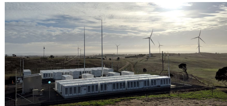
South Australia Battery at Lake Bonney, SA
