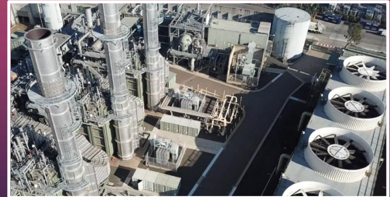
Smithfield Open Cycle Gas Turbine, NSW
