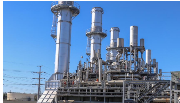
Smithfield Open Cycle Gas Turbine, NSW
