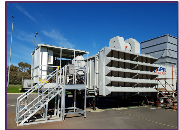
South Australia Gas Turbines
