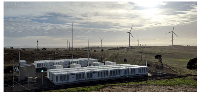
South Australia Battery at Lake Bonney, SA
