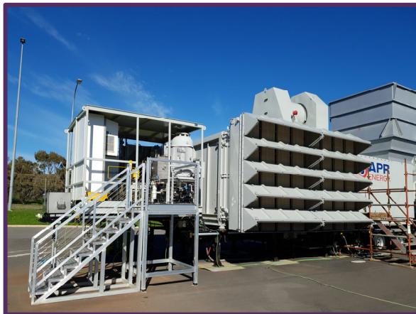
South Australia Gas Turbines
