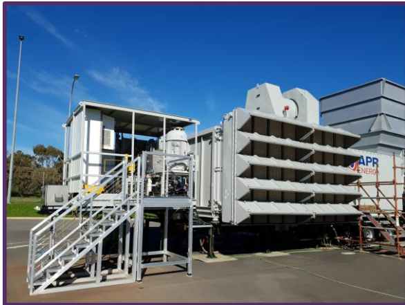
South Australia Gas Turbines
