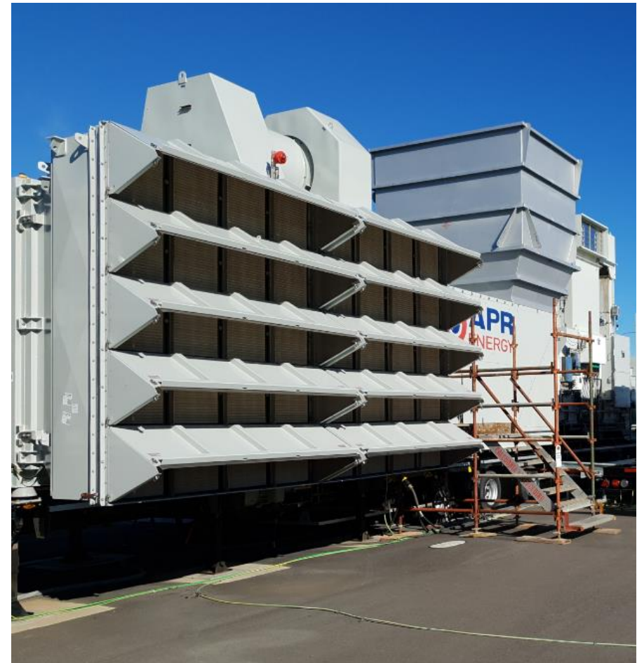
South Australia Gas Turbines, Lonsdale, SA
