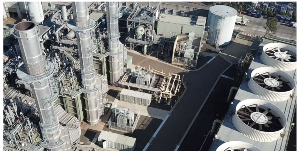
Smithfield Open Cycle Gas Turbine, NSW
