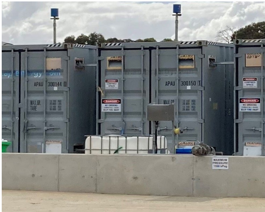
Figure 9: Fuel Storage and Fuel Forwarding Bund at BPS
