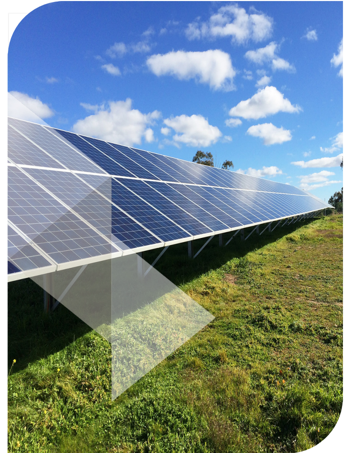
Capital East Solar Farm
