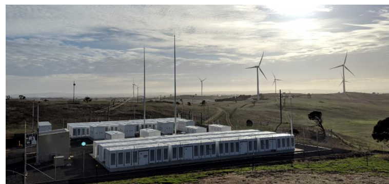
South Australia Battery at Lake Bonney, SA
